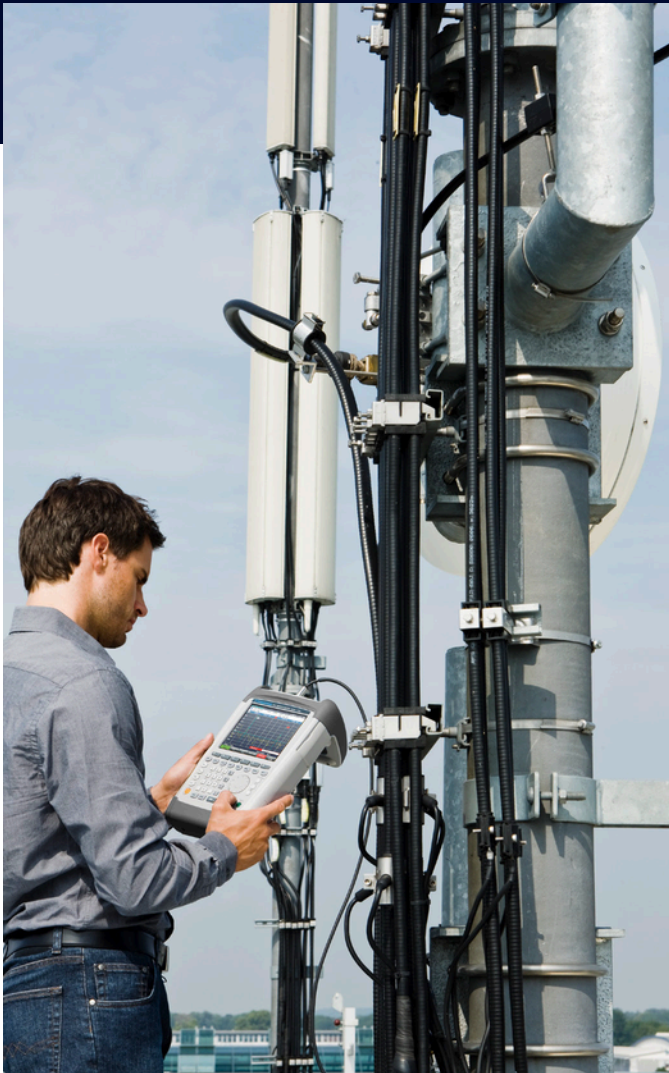
Distance-to-fault measurement at a mobile radio antenna system with the R&S®ZVH
